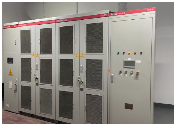
Install SVG dynamic reactive compensation device and capacitor cabinet to significantly reduce energy consumption
