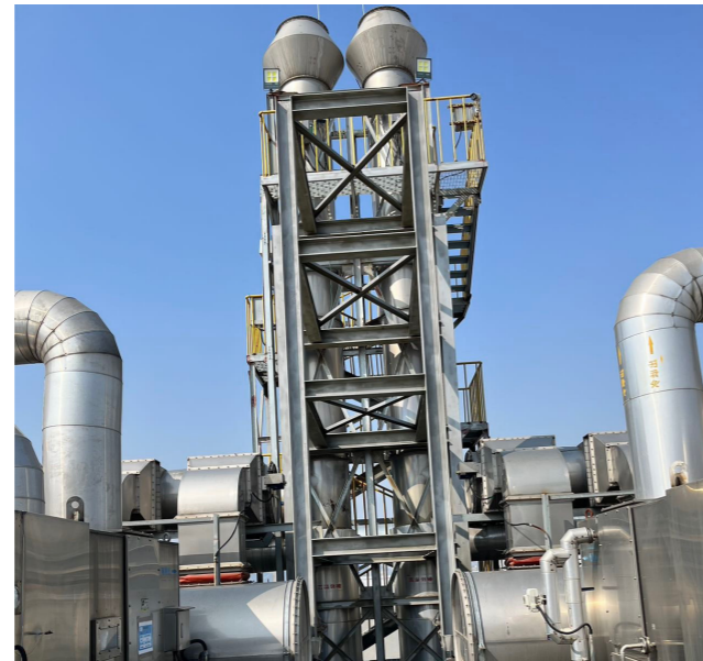
The VOC furnace temperature setting is lowered in a gradient to achieve a significant reduction in natural gas use while meeting VOC treatment standards.
