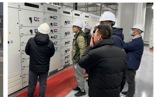
Staff regularly check the operation of equipment to investigate the potential safety hazards
