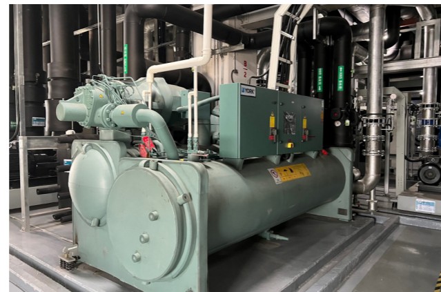
Hot water generated by chilled water heat pumps is used to supply ammonia and nitrogen wastewater treatment, significantly reducing the boiler turn-on time
