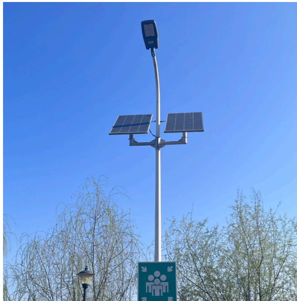
Upgraded solar photovoltaic street light
